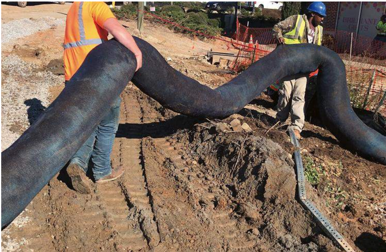
Silt sock filled with switchgrass are used at construction sites to control erosion. (MKB Company)
